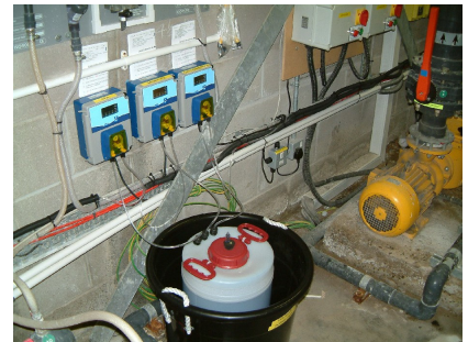
3 Dosing units serving 3 separate pools in Leisure complex, all fed from same day tank
